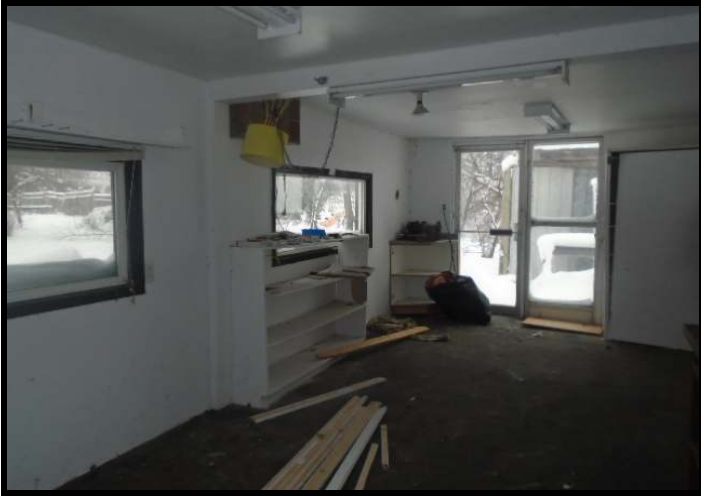
Insulation shop with gas line
