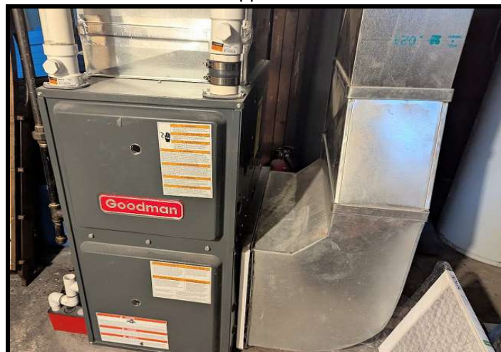
F/A Gas Furnace supplies main floor & bsmt
