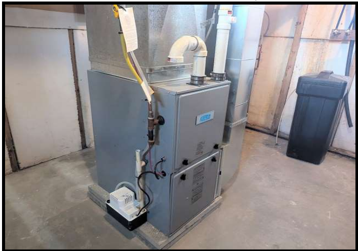
New Furnace in 2025 F/A Propane
