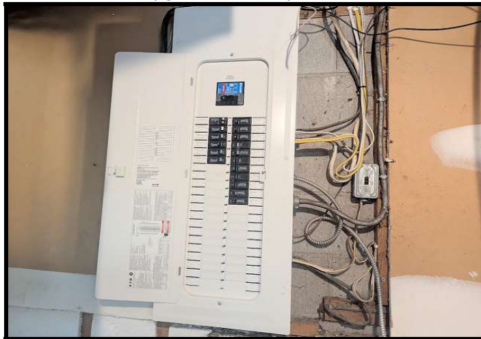
Upgraded 200 amp Panel
