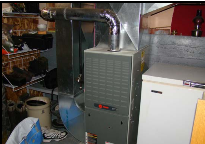
upgraded natural gas furnace
